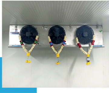
THREE FAN EVAPORATOR
