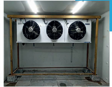
WALL MOUNTED BLAST CHILLER EVAPORATOR
